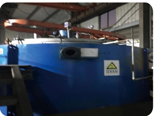
氮化炉 Nitriding Furnace
